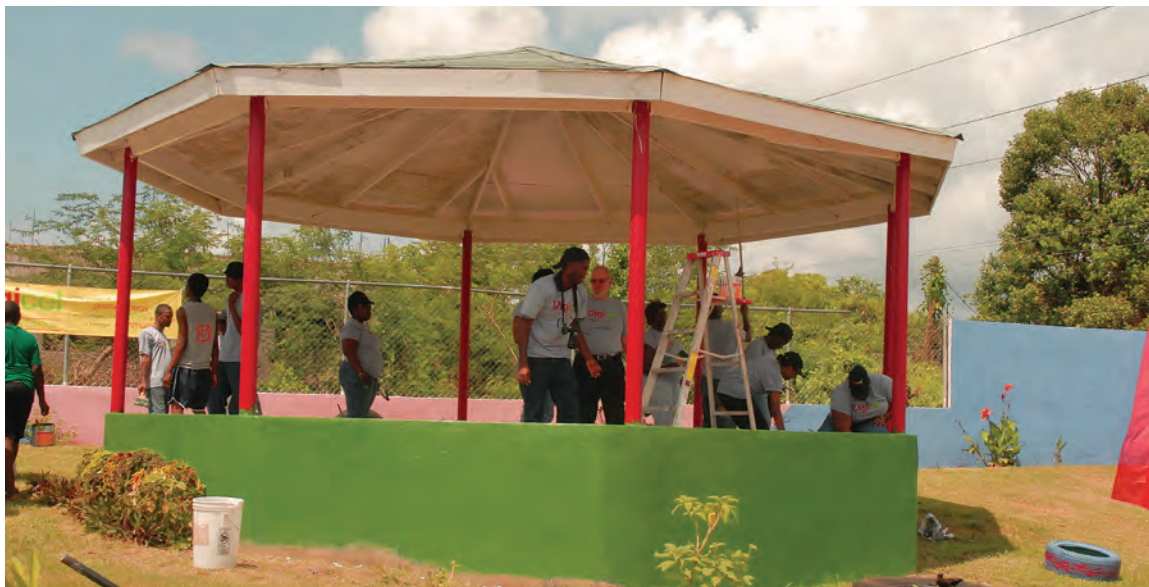
Putting finishing touches to the newly constructed gazebo in St. Jago South community
